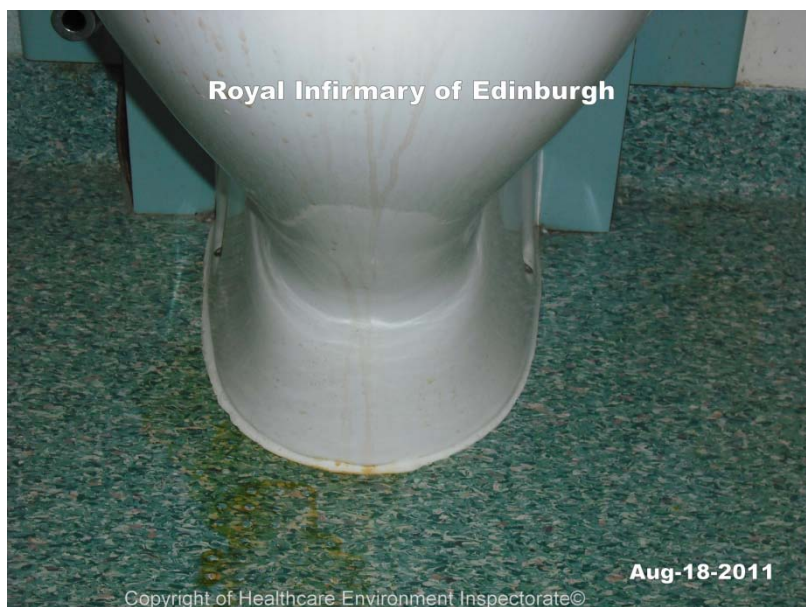
Image 1: Urine spillage in four-bedded bay toilet (ward 205)
